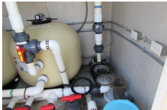
POOL PUMP and PIPING
